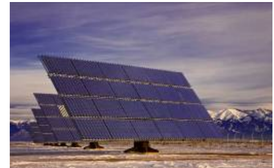
8.2 MW - Alamosa, CO Crystalline panels, fixed, one-axis, & dual-axis trackers, ground mount.
