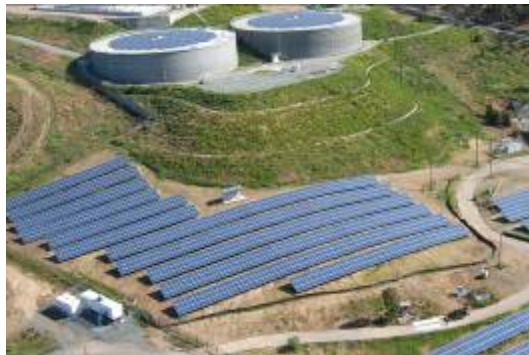
City of San Diego – Chula Vista, CA 944kW crystalline panels on tank top & ground mount
